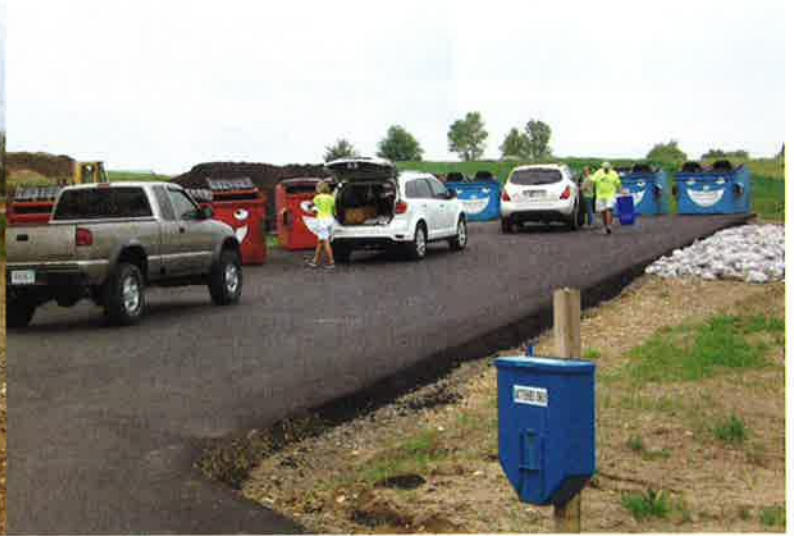
Completion of phase I of the Steuben Convenience Center. Phase II to be completed mid-August.
